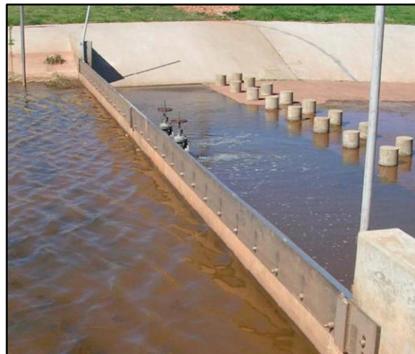
Photograph of Weir System on the South Diversion Ditch, Dyess AFB
